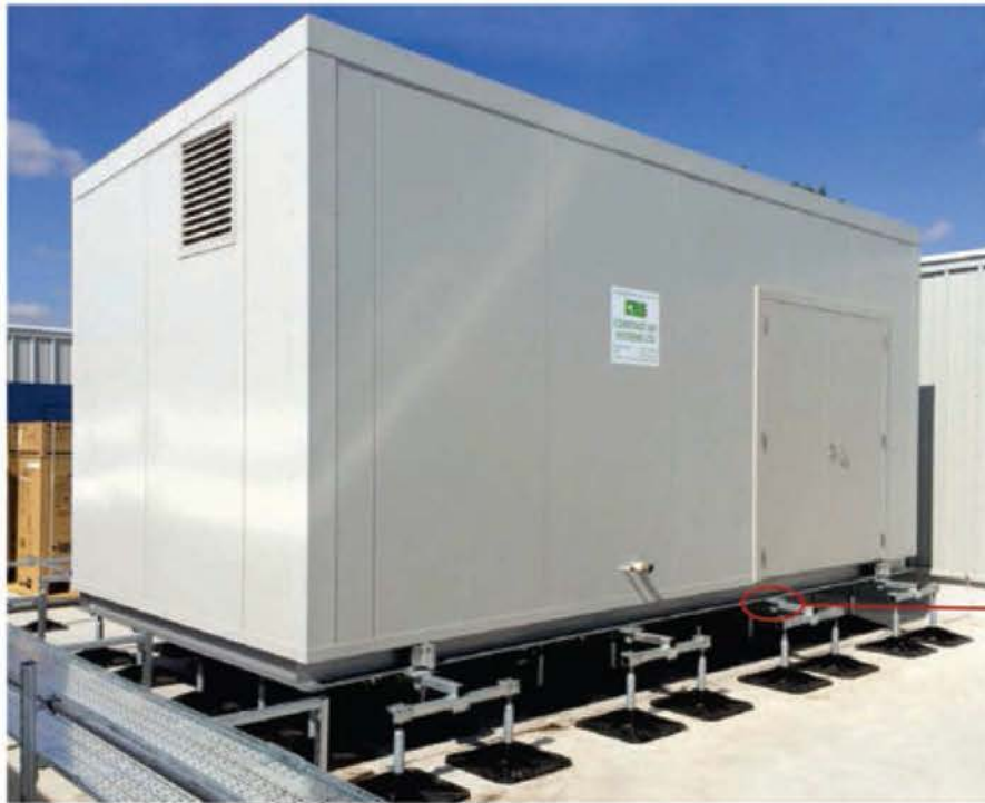
Typical plantroom support utilising 8no. F-QUAD-500-A
